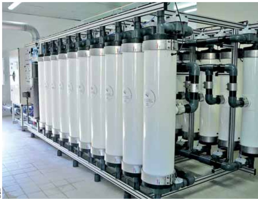
Ecoskid™ Aquasource Eaupotable 2000 m³ jour
